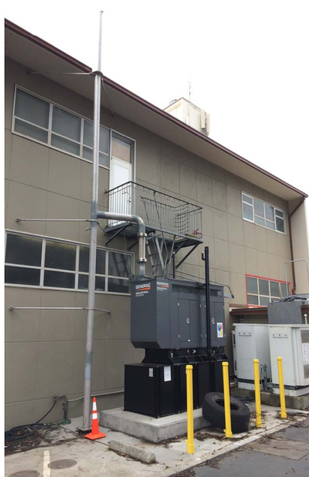
Station 15: New Emergency Generator
